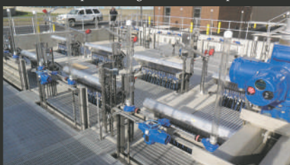
Bergen Point WWTP
